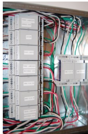
Power units are to be installed inside an enclosure.
